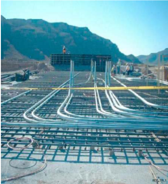
Significant underground installation of piping and electrical commodities, shown here at Silverhawk, helped reduce peak manpower loading.
