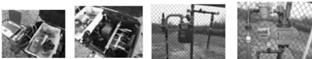
Test data collection , pressure regulation, redundant flow measurement (digital, mechanical)
