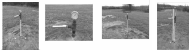
Pressure gauges and digital recorders at piping endpoints
