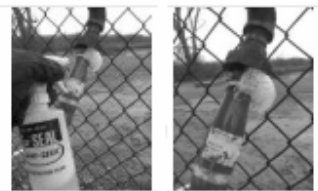
Leaks found during installation prior to repair and retest
