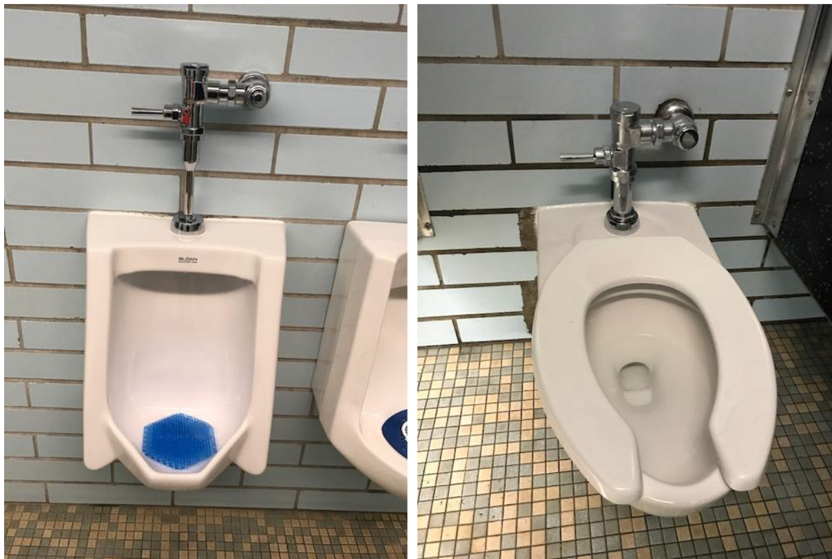
Figure 9 Water Efficiency Products installed at North Rockland High School
